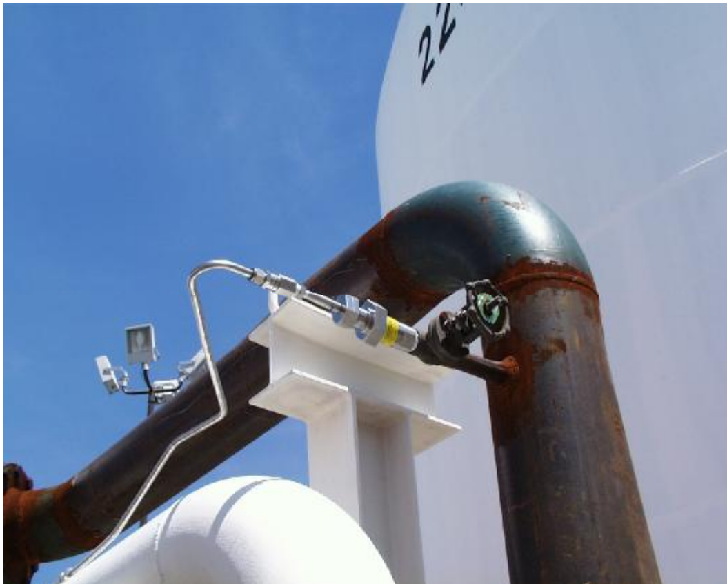
Figure 1 Typical Installation Courtesy of Seawaren, N.J.
