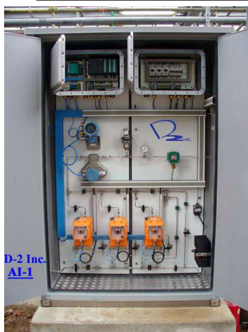
Open Skid Box (AI-1 w/ backup pumps)
