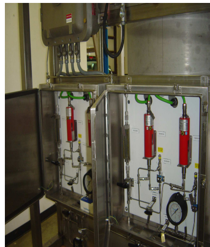
2 Diesel Line AI-1 w/ backups (Full Skid Shown on p.1)
